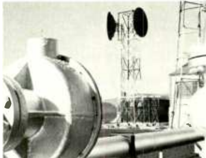
Mexican Pipeline Microwave System
